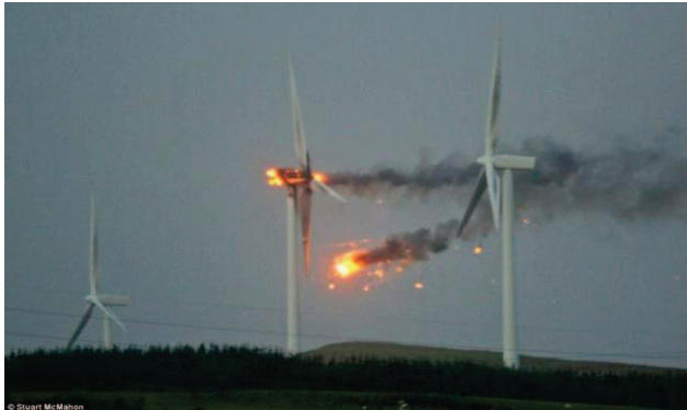
Wind Turbine Fire in Ayrshire Scotland
